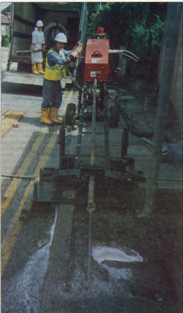
Terry Hackett and Sam Gardiner using the Jet Trac. Water cools the head and radio beacon, and assists cutting. In sandy soils additives can be mixed with the water to help support the bored-out passage until cable or ducting is installed, and a range of heads is available to cope with most types of ground. Earthing mats can be seen under and around the machine.
