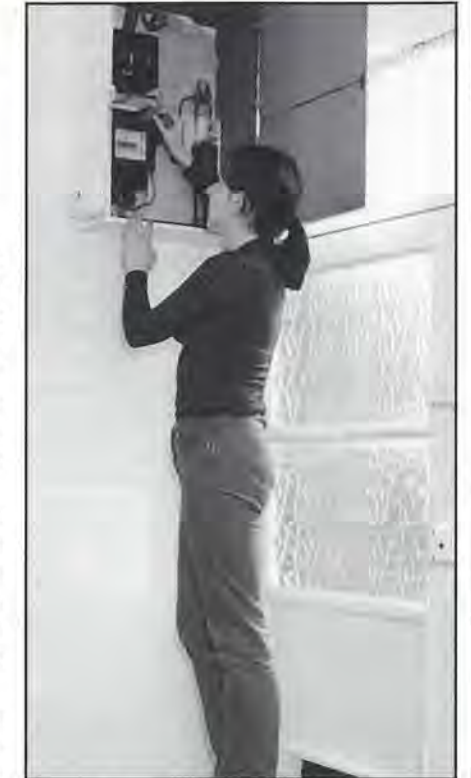
One aspect covered by the new Codes of Practice is that card meters installed in awkward positions - such as the one above - will be moved free of charge on request to an appropriate position for older and disabled customers.
