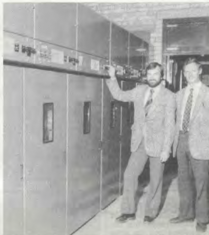
At a section of the 15-panel, 33-kV switchboard, we see Steve Chantler, left, and Dave Roberts.
