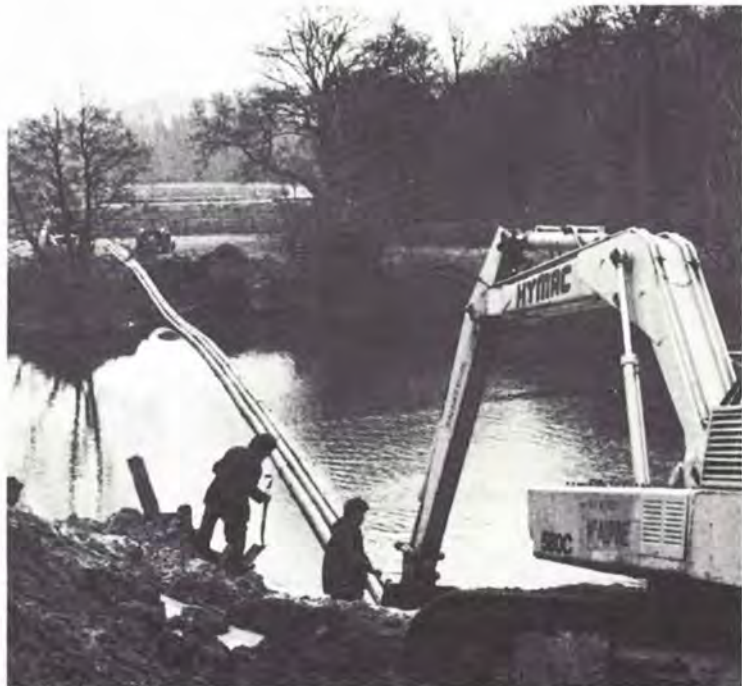
The PVC pipes, positioned across the water in readiness for sinking into the prepared trench in the river bed.
