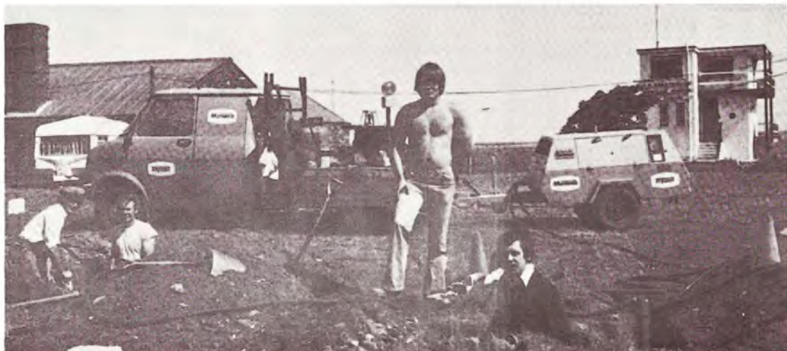
At Holyhead, as far West as you can go in the MANWEB area, our roving reporter came across a team of mains-men excavating a couple of very deep holes in the ground to unearth electricity cables. Our man learned that they were preparing to lay a new three-phase supply to the nearby coastguard station. Our picture, taken on one of the rare, warm and sunny days, shows the team, from left to right: Vivian Pritchard, Elwyn Jones, Robert Taylor and Dave Williams.
