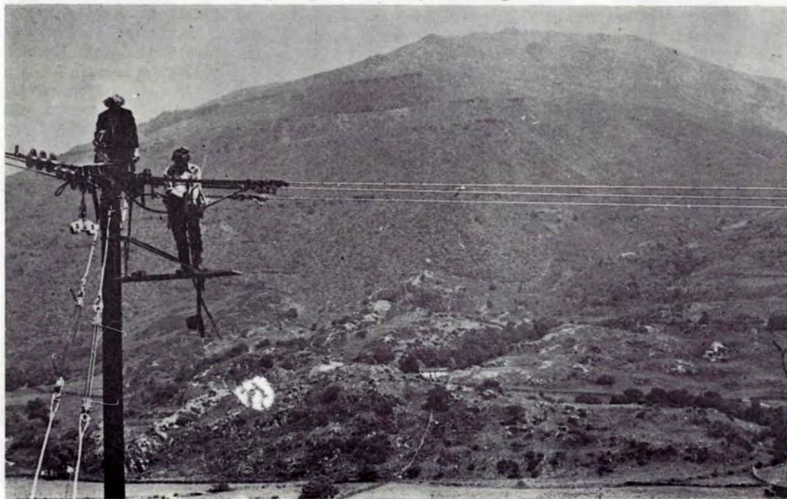
A new 11kV line, to supply power to the work-site at the upper reservoir, will climb the slate-heaps across the valley and pass over the skyline at a high level.
