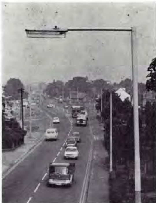
Photo-electric controlled street lighting on the A41 Chester by-pass.
