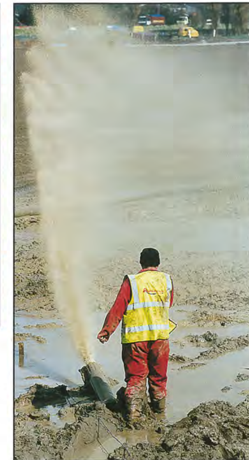
A successful outcome... the drill emerges on the far side of river bang on target, having laid the pipe below the river.
