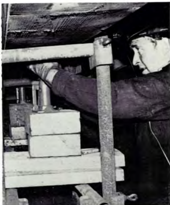
Mr. E. E. Davies makes a final check before the trough holding the cables is lifted.
