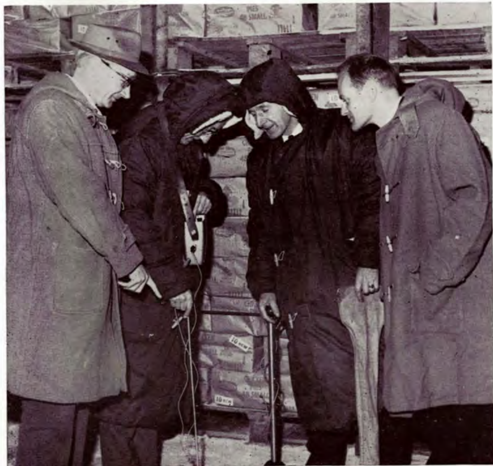
'That's the spot,' says Mr. K. Hill, left, (Electrical Engineer Birds Eye Foods Ltd.) as the men from MANWEB, Mr. Tom Owen (4th assistant engineer, Test and Development) and Mr. Jim Marland (contracting engineer), locate the fault in one of the huge ice-boxes. On the right is Mr. R. K. Pounder (Refrigerator Manager, Birds Eye Foods Ltd.)
