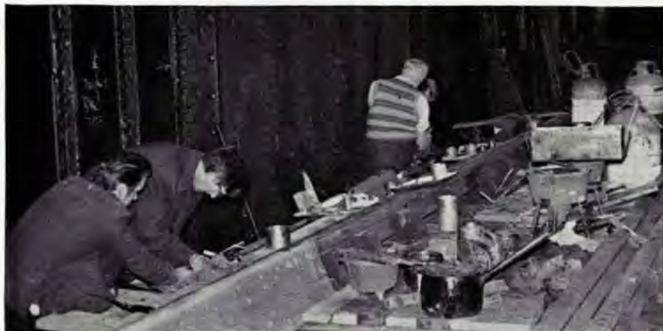
Engineering staff from our Anglesey District carrying out some 33,000 volt jointing on cable damaged by a train derailment.
